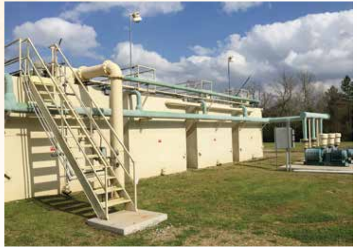
Aeration Basins and Blower
